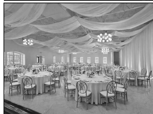
Carolina on Southport interior under renovation in late 2025 (top). The finished ballroom in March 2026, with a dance floor, seats 150-175 (above). Photos courtesy of Carolina on Southport.
