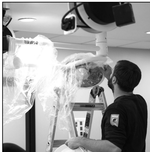
A worker puts finishing touches on the imaging room at the new Pet Resource Center.
